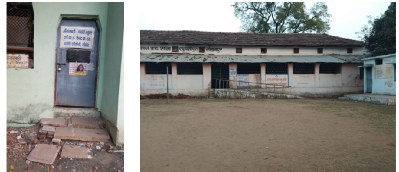
The water, sanitation and hygiene facilities at a school building in Madhya Pradesh.
